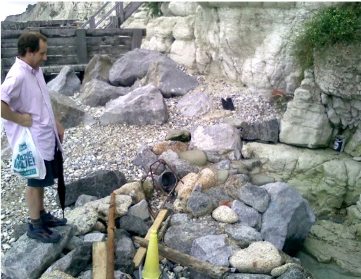
The 'Holy Well' - Hollywell, Eastbourne - a local citizen passing by observes the excavation work
